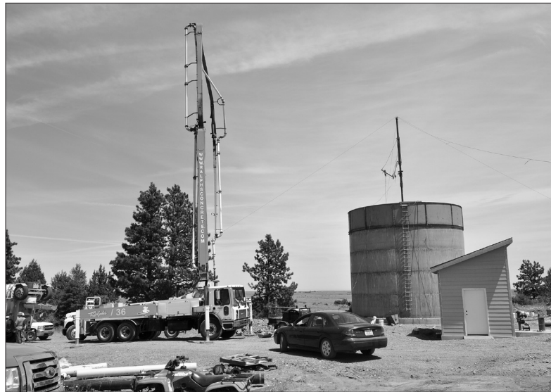
Building of the reservoir for Bickleton's new water system progresses in this photo taken Spring 2015.
